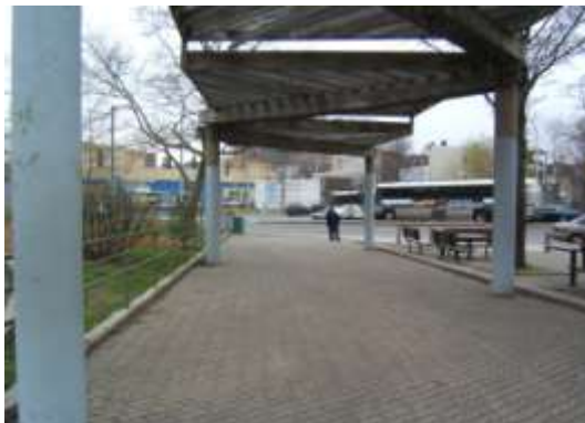
Figure 3 Deteriorated pergola over wide path
