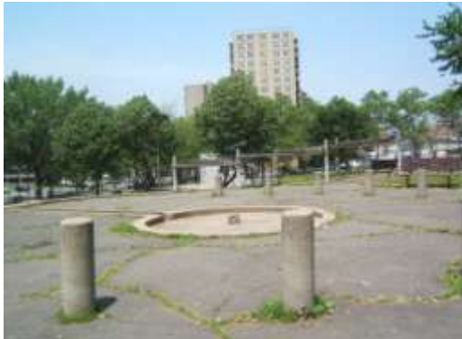
Figure 1 Asphalt around water feature, upper level
