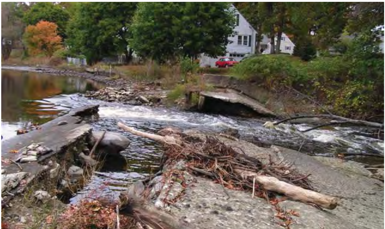
Figure 8.6 Damage to Winona Lake Spillway in Orange County on Quassaick Creek
