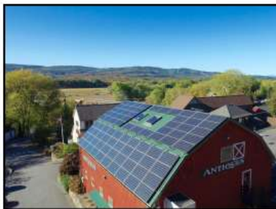
Water Street Market. Photo by Lighthouse Solar
